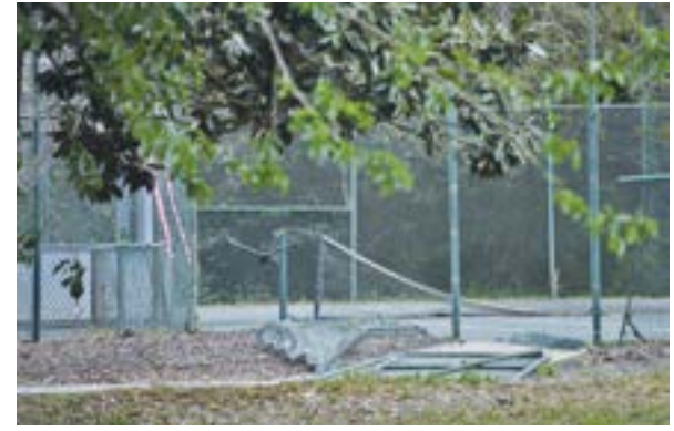
Fences are coming down at the Litchfield Racquet Club, which closed in October. Tanya Ackerman/Coastal Observer
