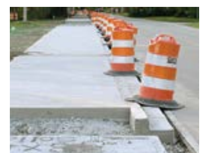
Charles Swenson/Coastal Observer Drainage work added to the cost of the path.
