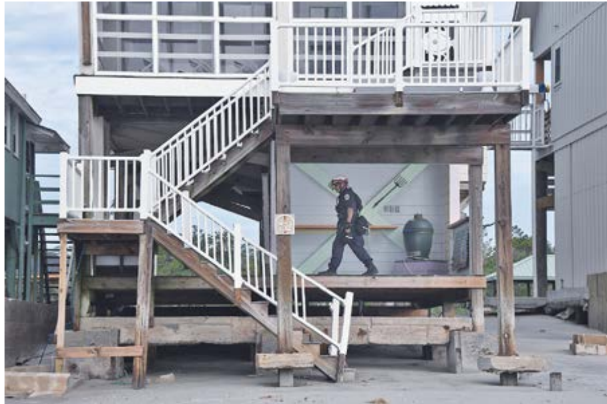
The storm scoured sand from under the foundation of a house on the south end of Pawleys.
